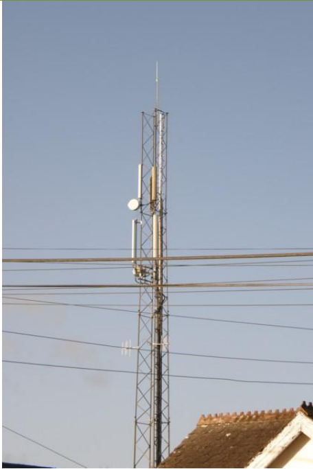
Transmitter Site Photo
